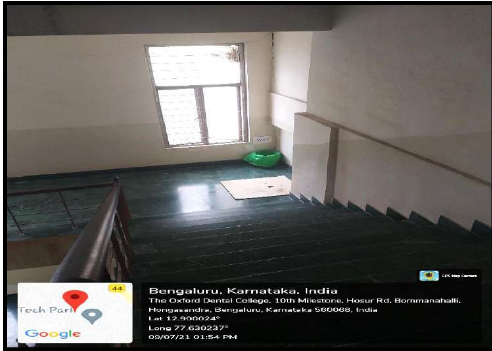
Dustbin in second floor Staircase
